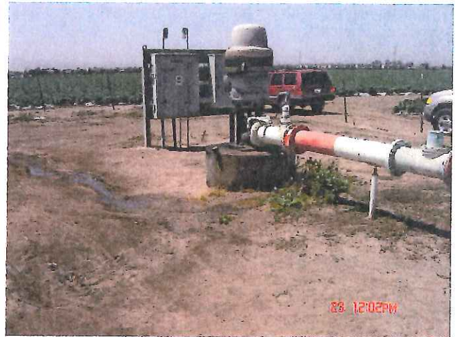
PHOTO 6: Looking south of de-sander towards irrigation well and electrical panel
