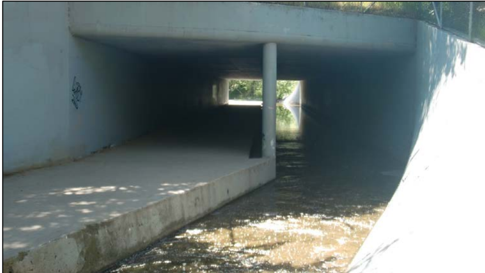
Figure 26 Looking downstream under Freedom Parkway bridge along Natividad Creek. The stream exits the valley bottom into a culvert for passage under the roadway. The stepped culvert provides additional floodway space during high flow conditions.
