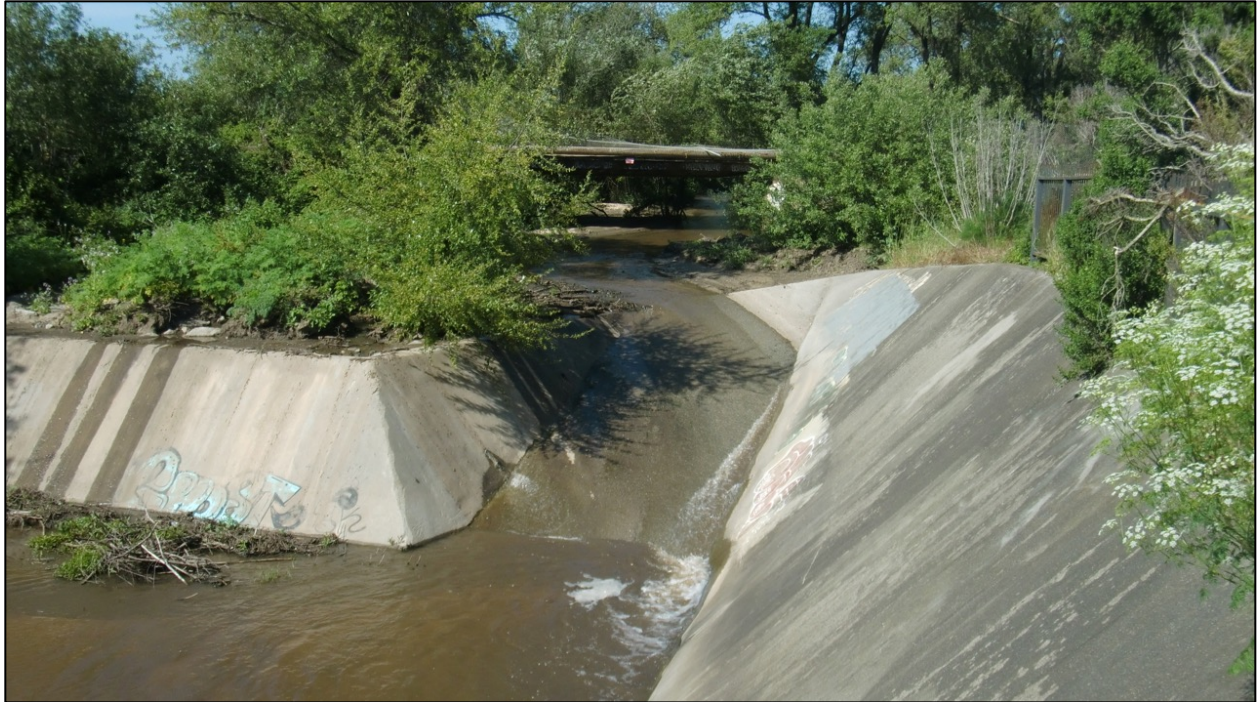
Figure 13 Looking upstream on Gabilan Creek at grade control structure, south edge of CASP project at Boronda Road and Independence Boulevard.
