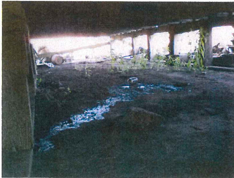
Photograph 4: View of oil puddle beneath Building B.
