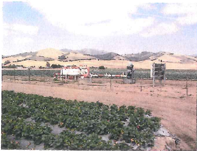
PHOTO 5: Looking northeast of site center towards irrigation well, de-sander, and electrical panel
