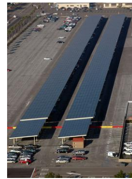
Solar Array at Coronado Naval Base
