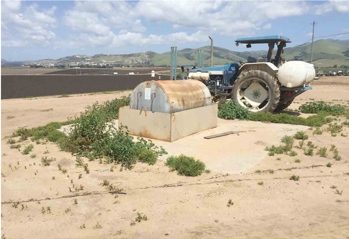
Photo No. 11 APN 153-091-012 – Diesel aboveground storage tank
