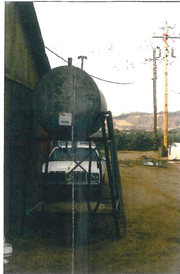
8. Parcel 4; Above-ground tank in ranch compound.
