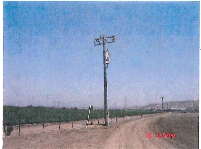
PHOTO 2: Looking north of site center, on-site electrical pole with transformer
