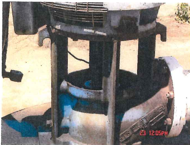
PHOTO 7: Close-up of irrigation well and running motor with fluid oil in the motor's reserve.
