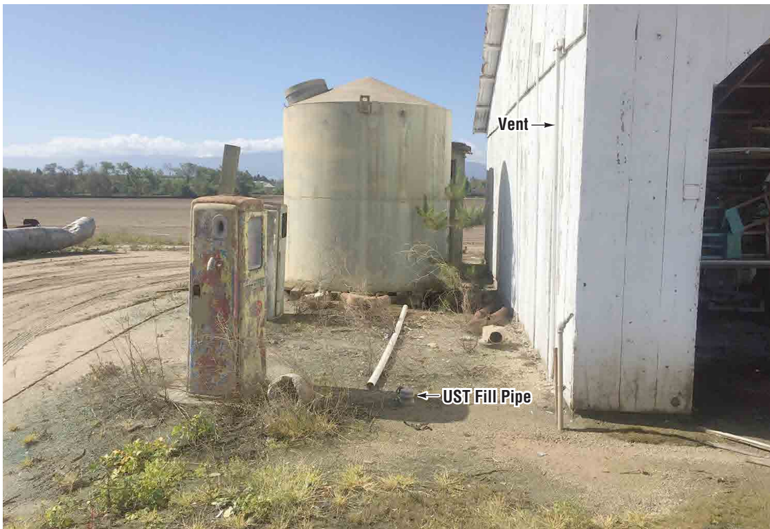
Photo No. 4 APN 153-091-001 – Abandoned underground and aboveground storage tanks
