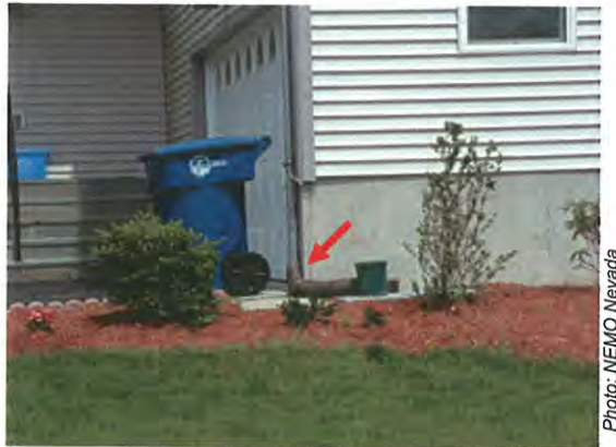
Figure 3-3: A Rooftop Downspout Redirected to a Landscaped Area
