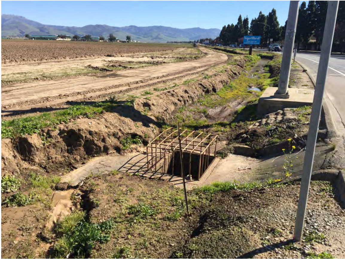
Plate 5 - Dartmouth Way storm drain inlet on the north side of Boronda Road
