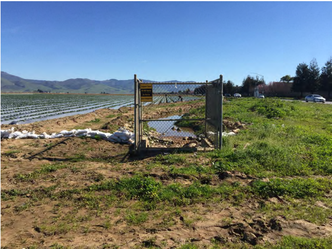
Plate 6 - McKinnon Road storm drain inlet on the north side of Boronda Road
