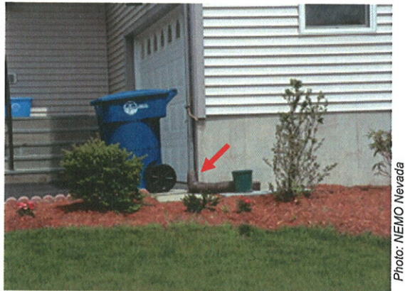
Figure 3-3: A Rooftop Downspout Redirected to a Landscaped Area
