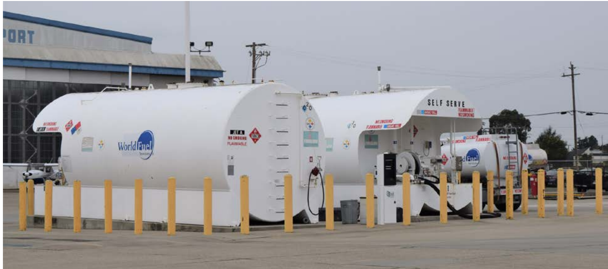
Figure 1.23 – World Fuel/Jet West Fuel Farm
