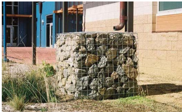
Gabion for Energy Dispersion (i.e., erosion control)
